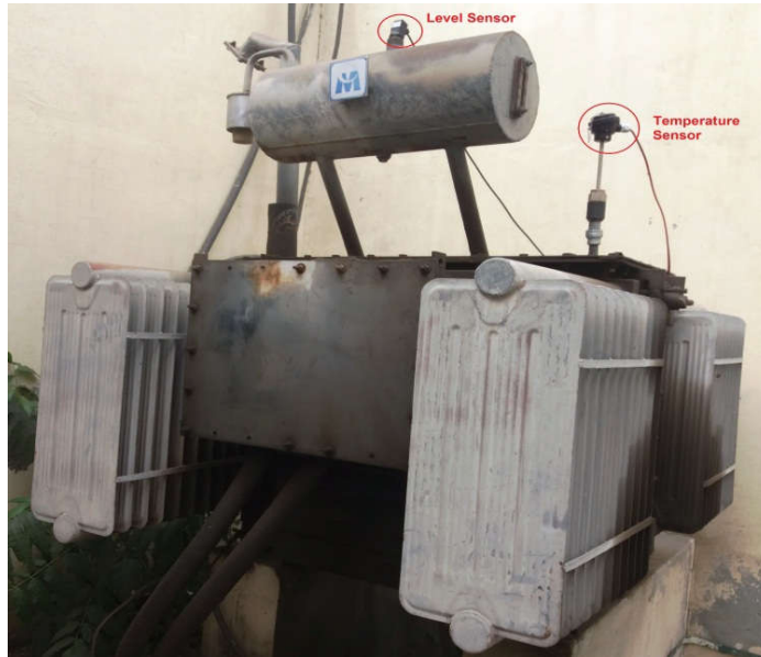
Figure 4.1 400 KVA Distribution Transformer used for online monitoring
