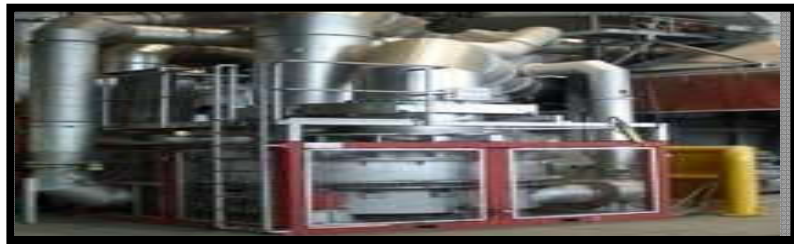
Figure 3.5 Rotary Regenerator on a Melting Furnace
