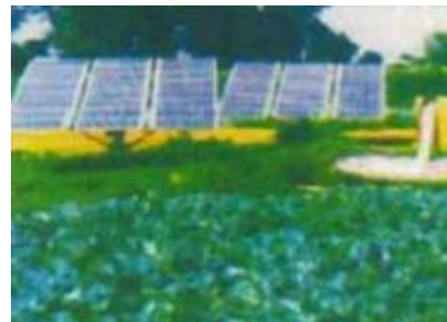
Fig. 9: Solar water pump
