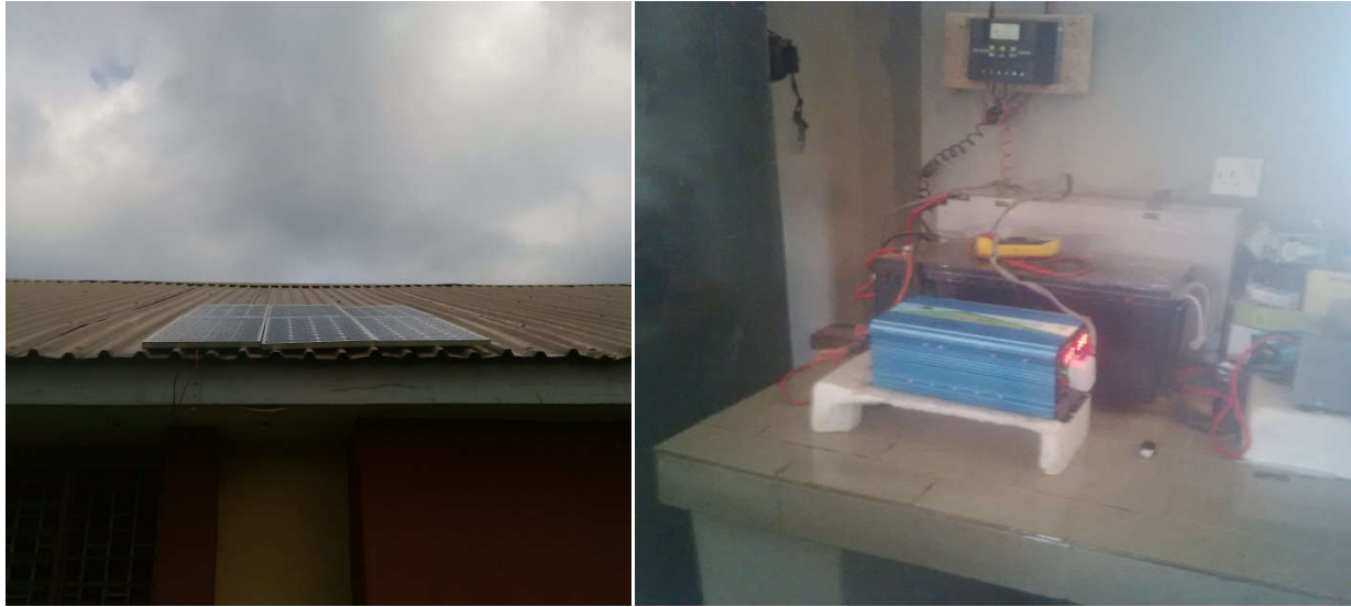
Plate 2: The view of the installed six 80 W (480W) solar panels, CM 5024 PWM 40 A digital intelligent solar charge controller 12/24V, 400 AH solar batteries and the 2000 W solar inverter used for the laboratory investigation.
