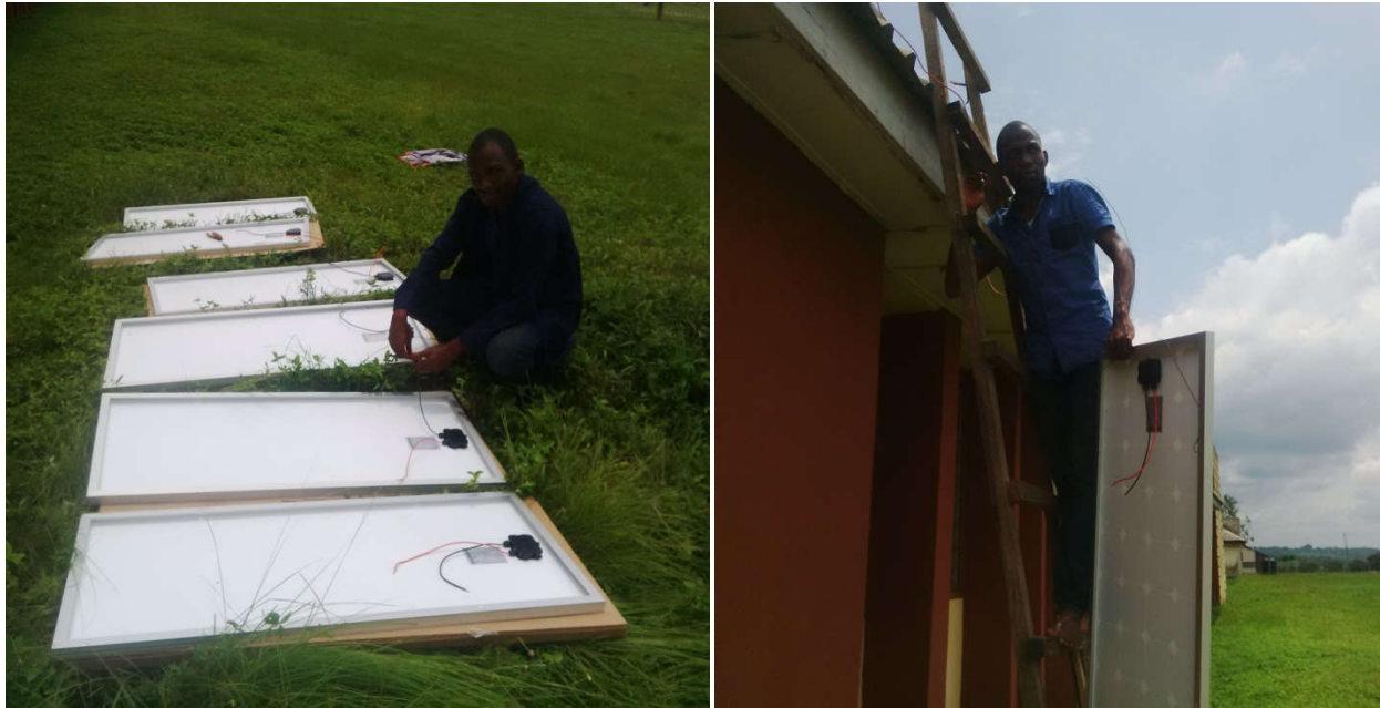
Plate 1: The views of the six 80 W (480 W) mono-crystalline photovoltaic solar panels during field investigation and installation.
